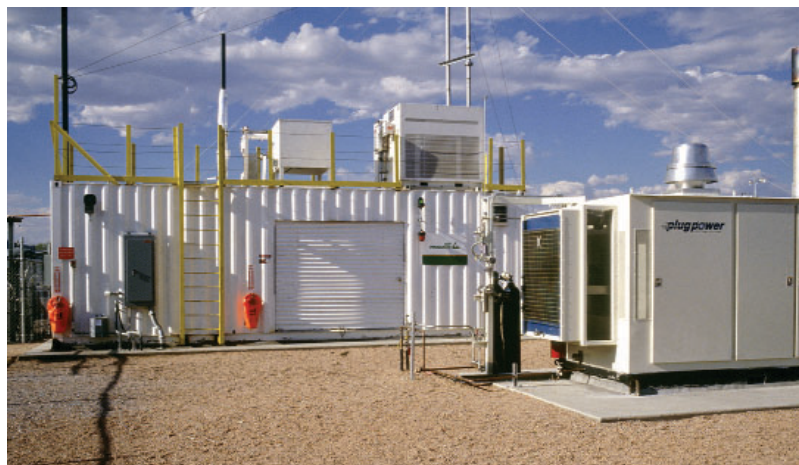
The Las Vegas Energy Station, where a hydrogen generator (left) installed by Air Products and Chemicals, Inc., produces hydrogen through the reforming and purification of natural gas. This hydrogen fuels vehicles and Plug Power's PEM (proton exchange membrane) fuel cell (right), which provides electrical energy to the Las Vegas grid.
